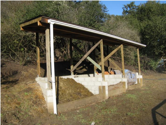
Three Bin Manure Bunker System
