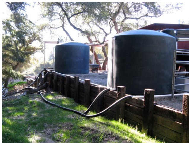
This rain catchment system collects water from roof and gutters and stores it for future use or for slow release after the storm.
